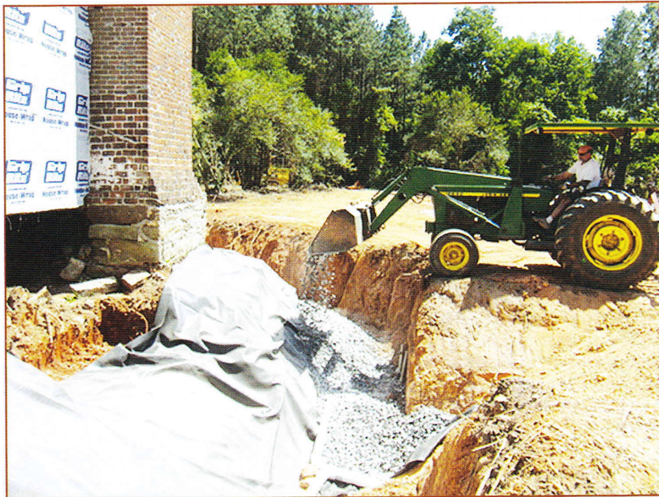
King using the tractor to fill the drainage ditch for the waterproofing system with rock.
